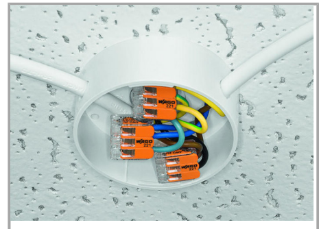
Lighting distribution in ceiling canopy
